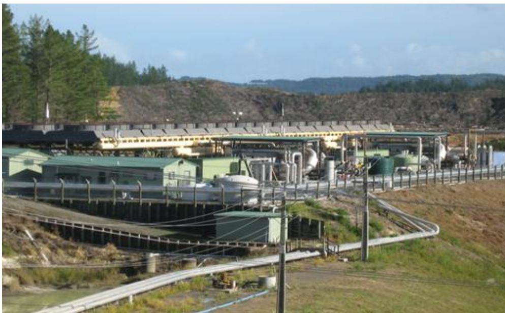
Station 1: 10MWe Ormat binary plant commissioned in 1998
