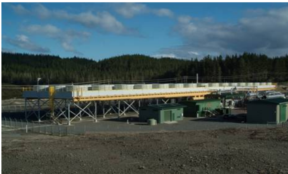
Station 2: 15 MWe Ormat binary plant commissioned in 2008
