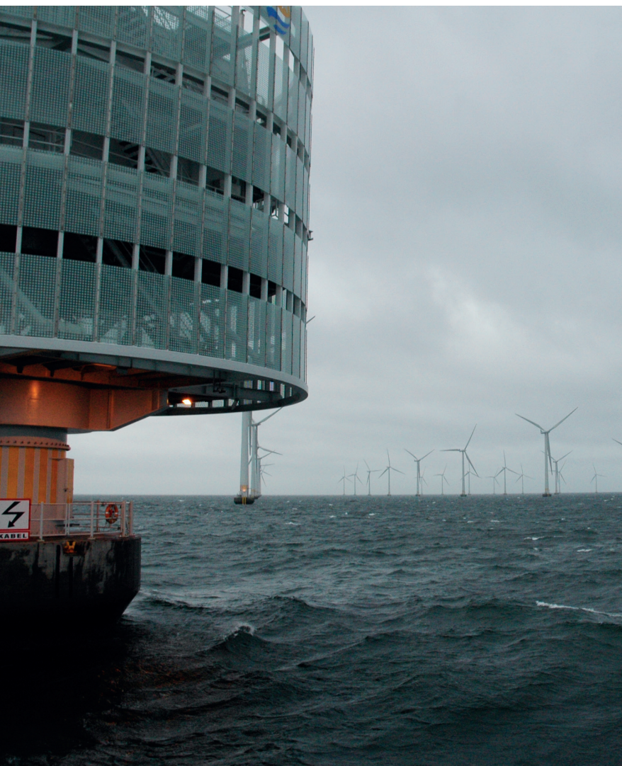
Offshore wind turbines (Denmark) with substation in the foreground
